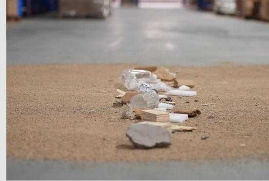
Dust & debris affecting machinery & goods
